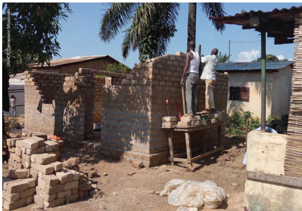
Building houses to support returning communities in Bangui, Central African Republic, in 2017.
